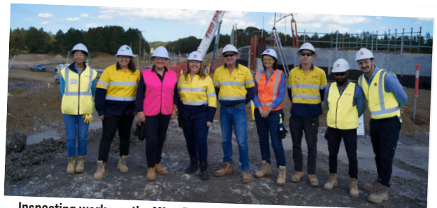
Inspecting works on the M1 to Raymond Terrace with Federal Member for Paterson Meryl Swanson.
